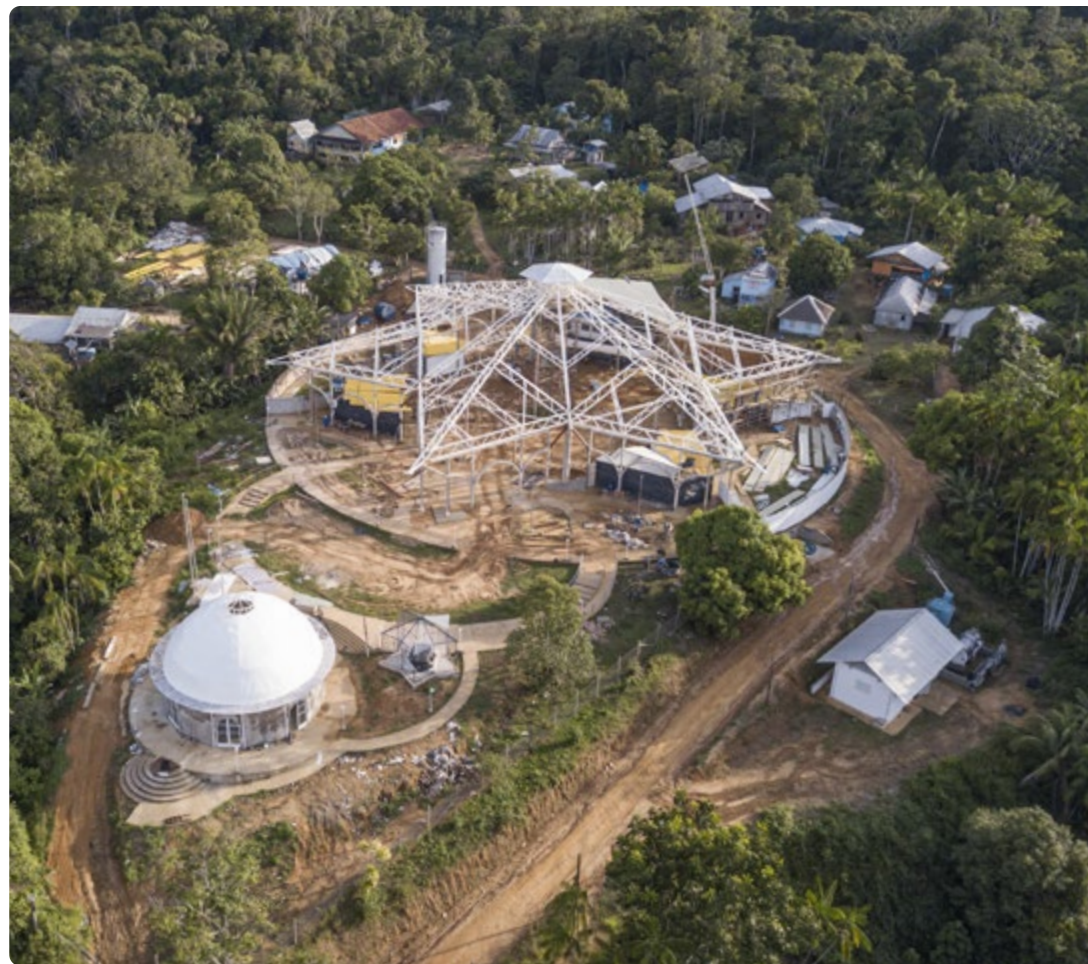
Aerial photographs of the final stage of construction – installation of the metal roof structures. Photos: Iberê Périssé
