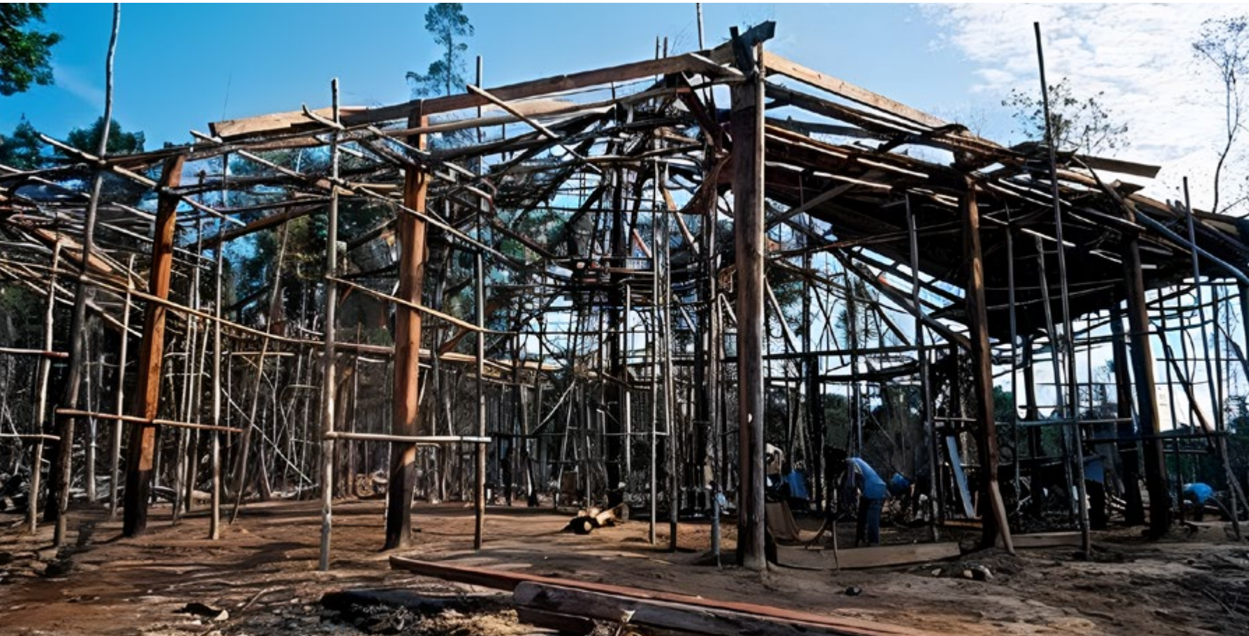
Construction of the old church in the late 1980s, using local timber and labor. Photo: Acervo CEDOC.
