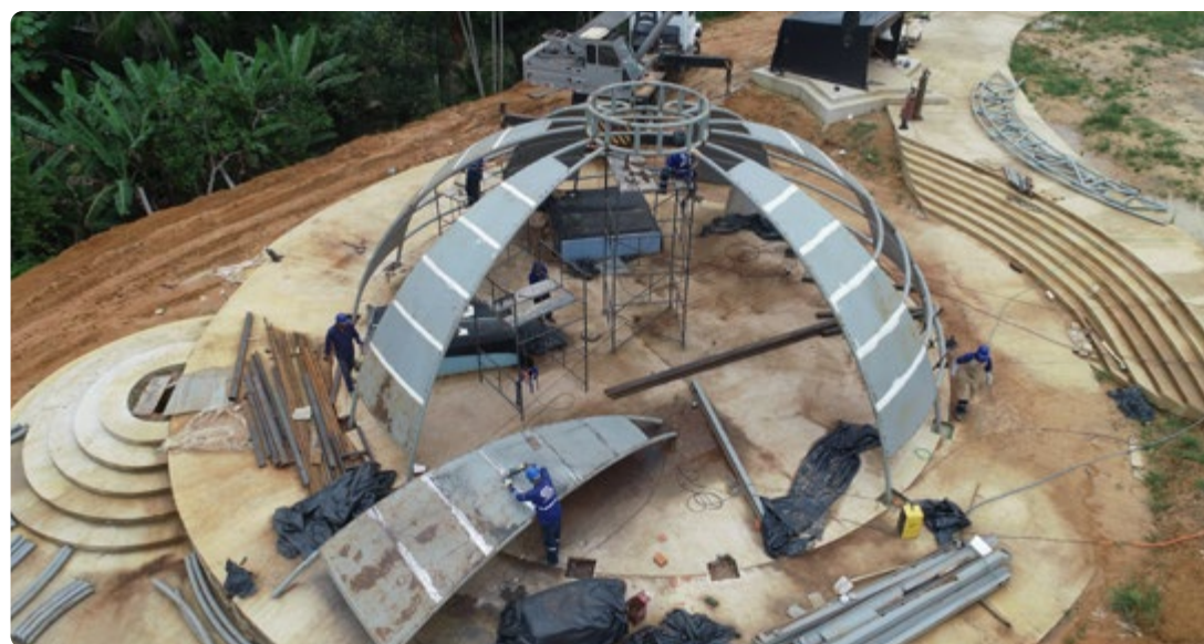
Aerial photographs of the construction stages of the Padrinhos' tombs and the masonry structures in the main hall. Photos: Pedro Adnet
